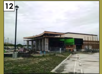
12 Collin College Conference Center 2200 W. University Drive Valuation: $4.6 million Permit Issuance: August 2014
