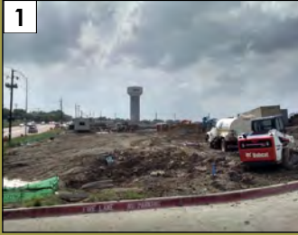
1 Walmart Neighborhood Market & Fuel Station 3400 Virginia Pkwy. Valuation: $4.1 million Permit Issuance: April 2015
