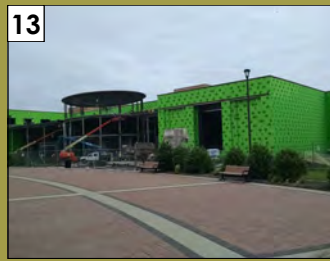
13 Collin College Health and Sciences 2200-A W. University Drive Valuation: $25 million Permit Issuance: July 2014
