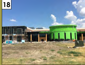
18 Collin College Health and Sciences 2200-A W. University Drive Valuation: $25 million Permit Issuance: July 2014
