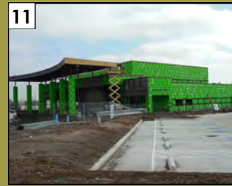
Collin College Conference Center 2200 W. University Drive Valuation: $4.6 million Permit Issuance: August 2014
